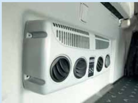
Quickly done: installation of the evaporator unit at the inside rear wall of the cabin.
